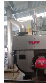
Installed biogas boiler
