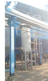
De-aerator system – to remove H 2 S
